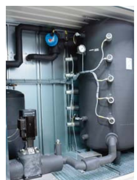
Hot water- tank
