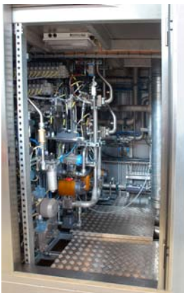
Walk-in hydraulic rooms
