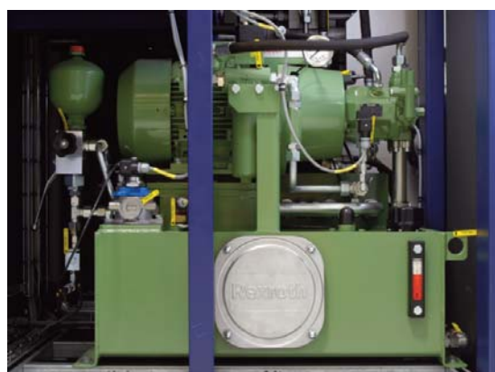
Hydraulic power unit
