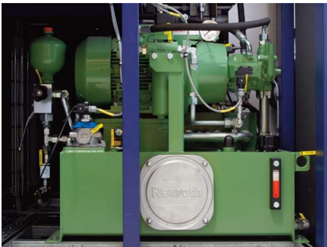
Hydraulic power unit
