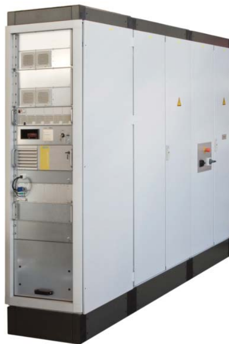
Switch cabinet and control console
